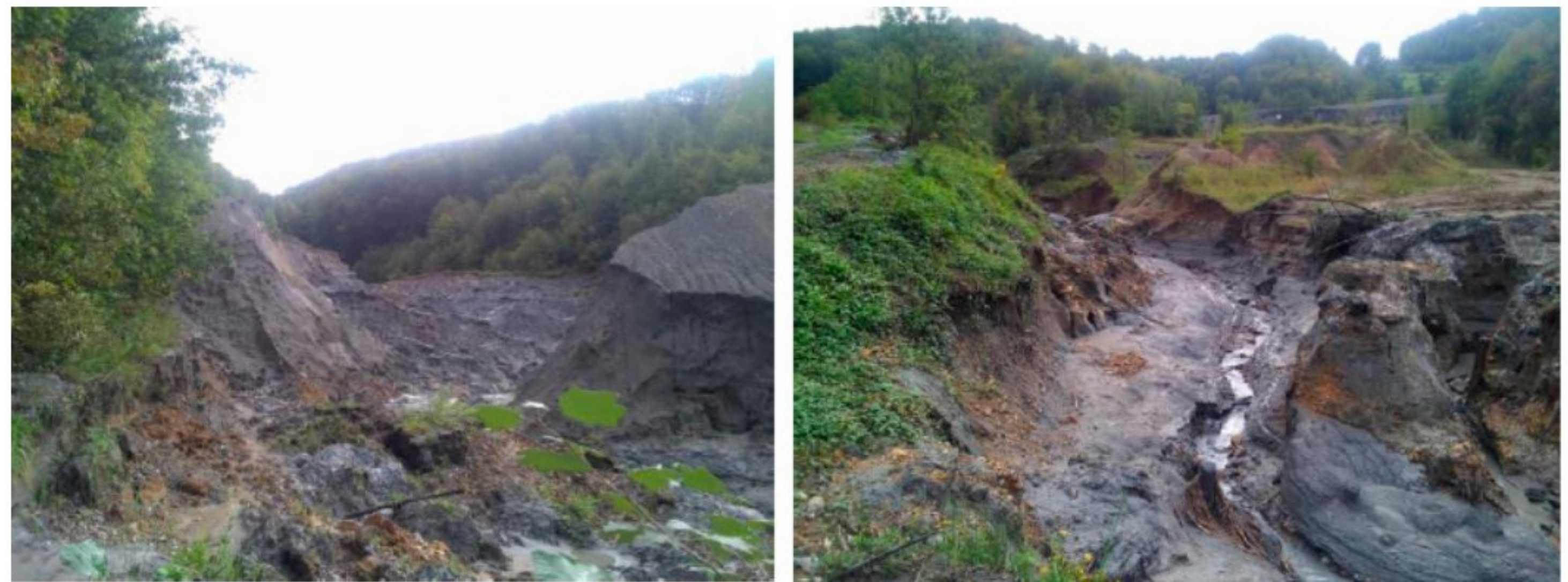
Figure 4. The damaged embankment of the eastern field. Reproduced with permission from the Water Institute “Jaroslav Černí” [10].
