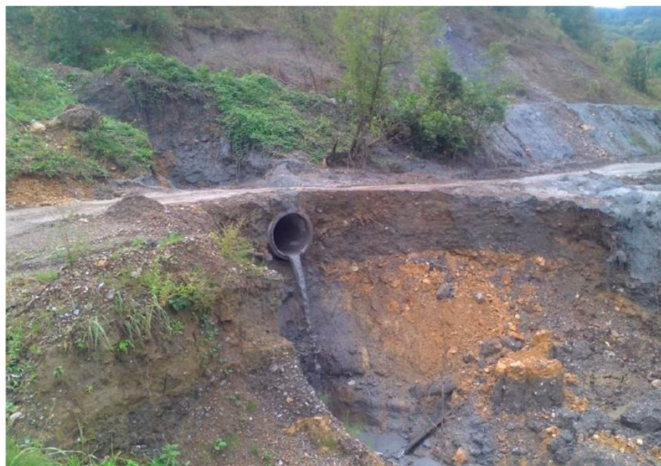
Figure 5. The damaged pipe culvert on the western field. Reproduced with permission from the Water Institute “Jaroslav Černí” [10].
