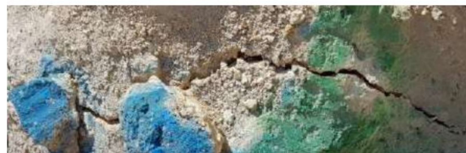
Figure 8 Crack formed by the action of expansive mortar [7]
