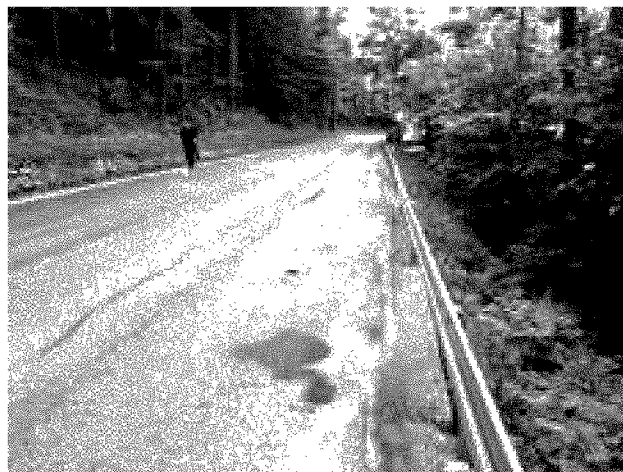
Figure 2 Photo of the state road DC3 (section 015) at km 2+060 before remediation works. Tension cracks at the crown of the landslide Dedin are visible on the asphalt.
